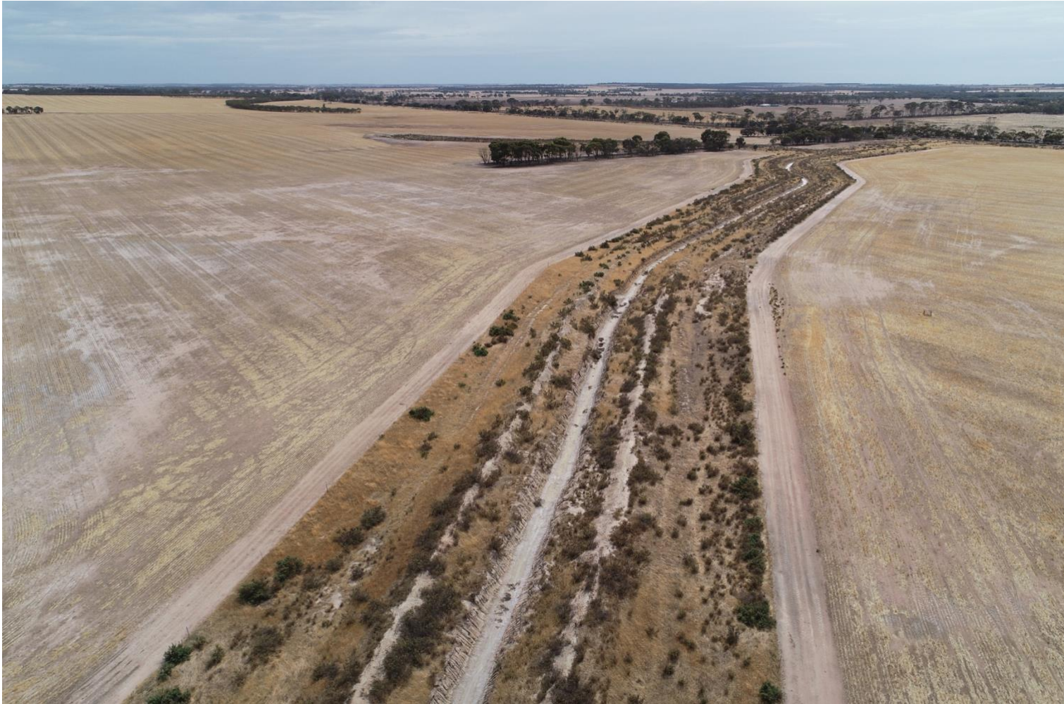
52km of drains stretch across the Dumbleyung landscape in the Fence Road Arterial Drainage Scheme.
